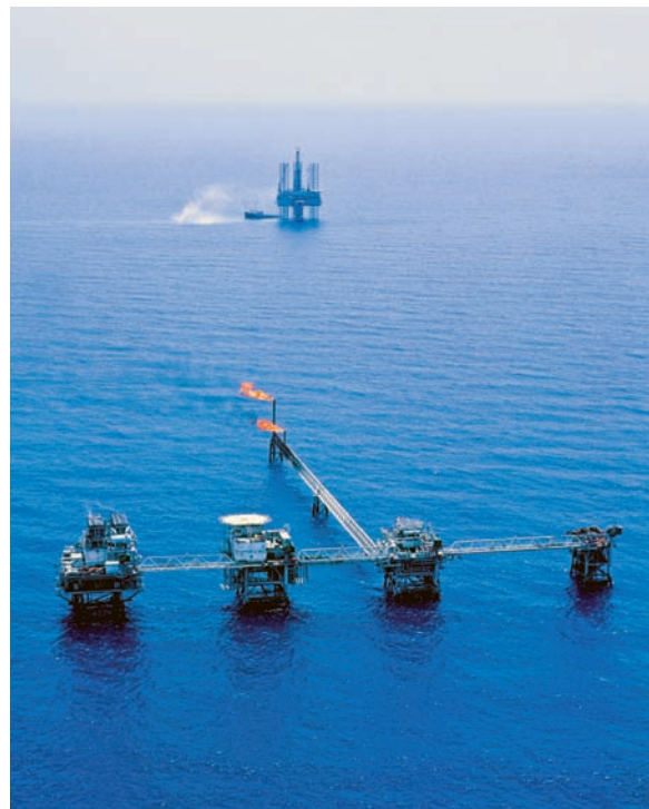
Figure 5.2. Offshore production platform with jackup drilling rig in background
