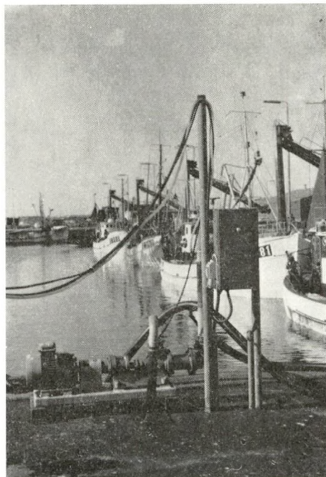
Fig. 5. Pump for bilge water.
