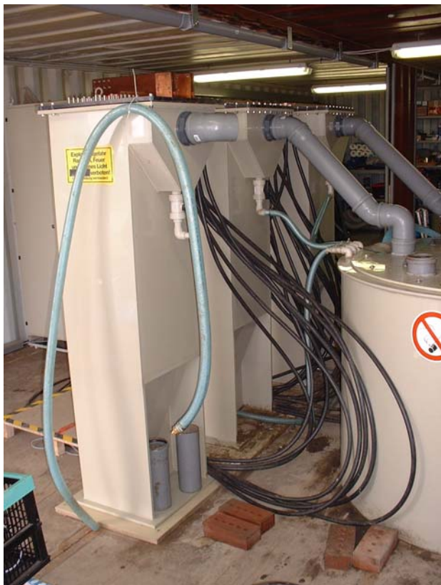
Figure 6.13. Electrolysis cells of the TU Harburg plant.
