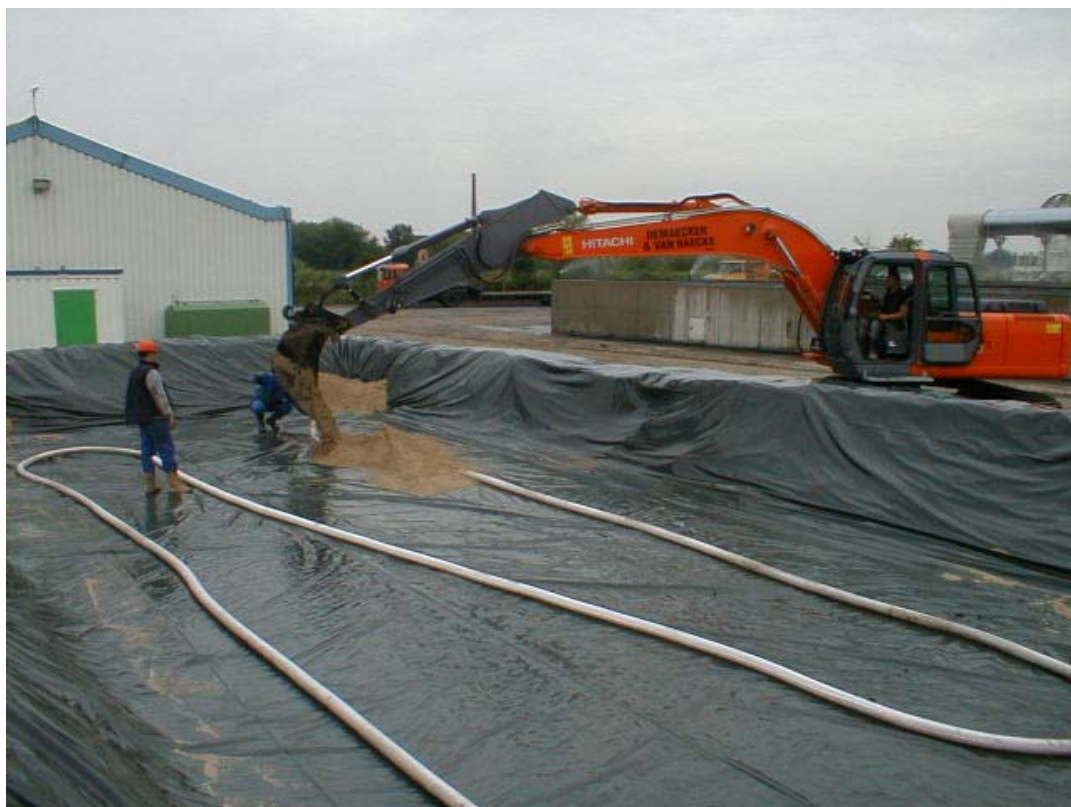
Figure 2.5: installation of the lagooning fields: view on welded liner and drainage collection pipes.
