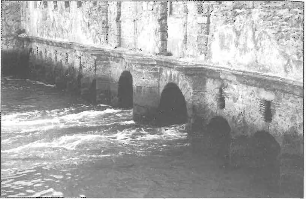
Fig. 11. The main façade of the Arillo Mill (Cadiz, Spain). Water flowed into the pond through eight entrance sluices: four on main façade and four others perpendicular to the mill (not seen here); the most important are behind the two larger central arches. All the exit sluices are on this main façade. (Photo Loïc Ménanteau, November 1991).
