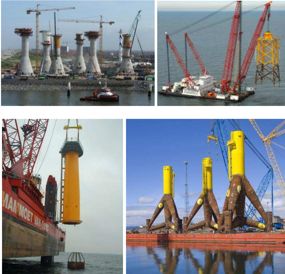
Figure 2. Typical Fixed Support Structures: (a) GBS (Thornton Bank.1. Source: C-Power). (b) Jacket (Thornton Wind Farm. Source: C-Power). (c) Monopile (Princess Amalia. Source: belwind.eu ). (d) Tripod (Alpha Ventus. Source: Alpha Ventus)
