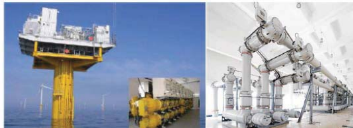
Figura 60 - GIS offshore substation (Alstom, at left) Indoor GIS substation (ABB Elk-3, right)
