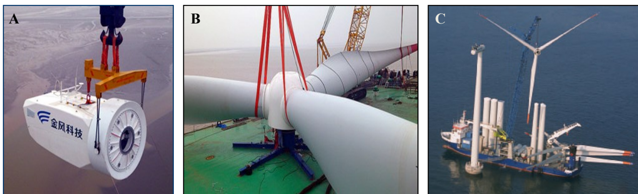
Figure 2.10 Lift of the nacelle with a generator (A). Assembled rotor on-board the vessel (B) and lifting of the rotor with the blades pre-attached (C)
