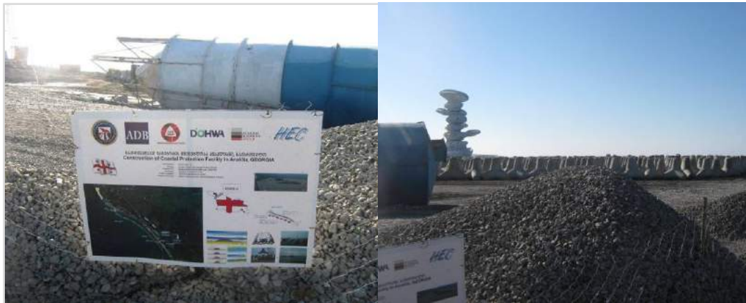
Figure 10: ADB is supporting the project for the arrangement of 10 tetrapod breakwaters, placed at 250-300 meter inshore of the beach along 4.1 km length of coastline. The cost of 1 st stage is approx. EUR 6 million, 2 nd estimated at 4-6 million
