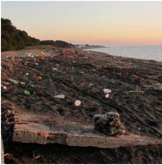
Figure 23: Concrete fences collapsed, southward view at Tskaltsminda coast. Best intervention would be regular beach litter cleanup
