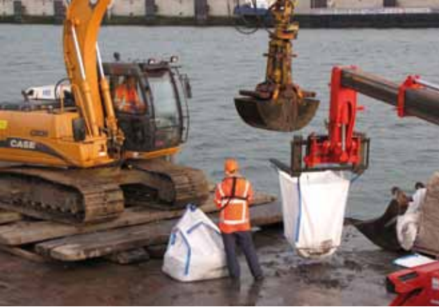
Fig. 2.21. The backhoe divided the soil from the container over two bulk bags, A and B.
