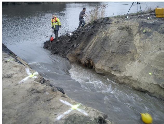
Figure 6-1 Floats in breach
