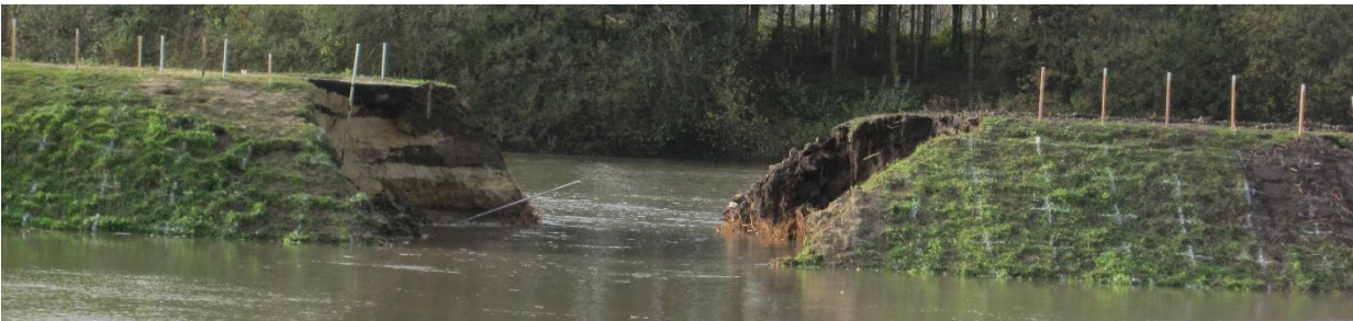
Figure 5-5 Breach after day II photographed from the polder 17/11/2015
