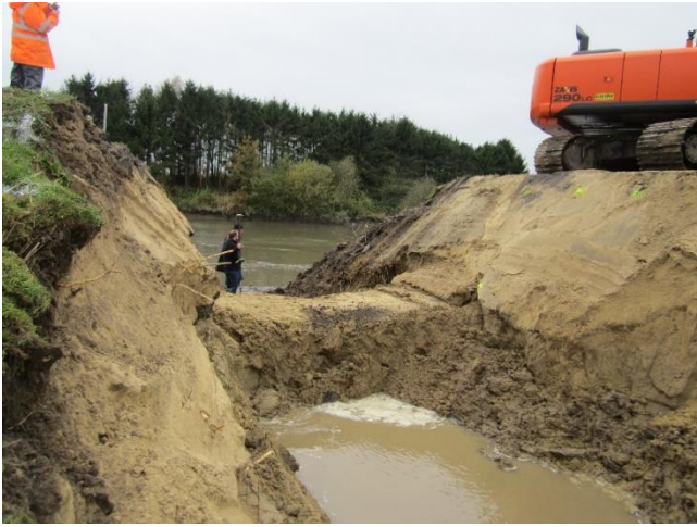
Figure 5-2 Breach after breach test I 16/11/2015
