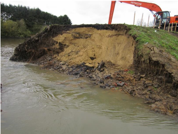
Figure 5-3 Breach during test II 17/11/2015
