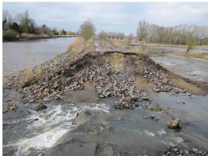
Figure 5-11 Inside of the breach 8/02/2016
