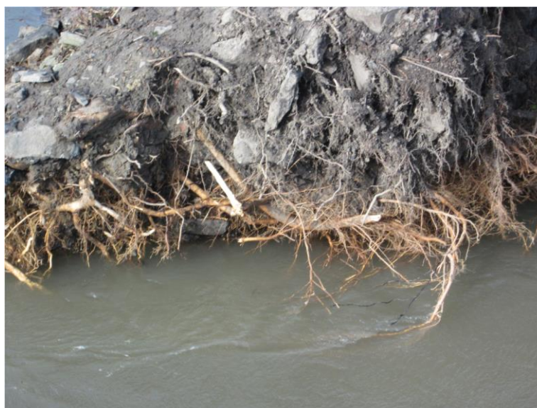
Figure 8-7 Roots in clay lining
