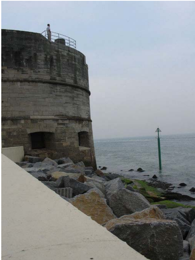
Figure 9.9 Modern coastal protection works employed at the base of the Round Tower, Portsmouth
