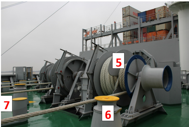
Figure 2.12: Overview mooring equipment (II), (5) winch, (6) roller guide, (7) bitt.
