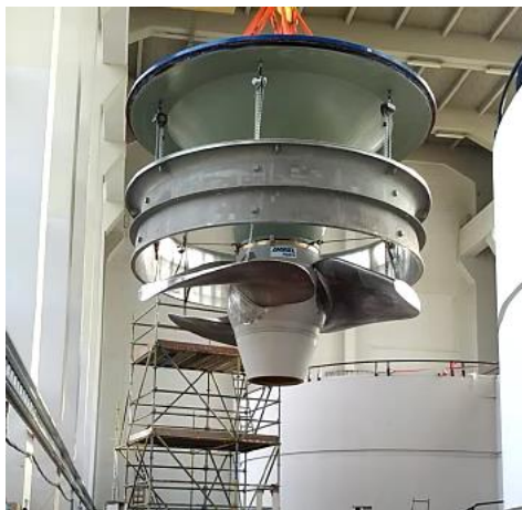
Figure 4: New eco-sustainable turbine at Monsin HPP
