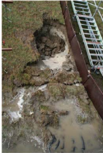
Figure 26: Final result St Philipsland, Zeeland. Damage to the rear side at the maintenance road, which started at 30 l/s per m. Removal of the whole maintenance road. Picture taken half way the 75 l/s per m test. The hole became at the end 15 m wide and about 1 m deep.
