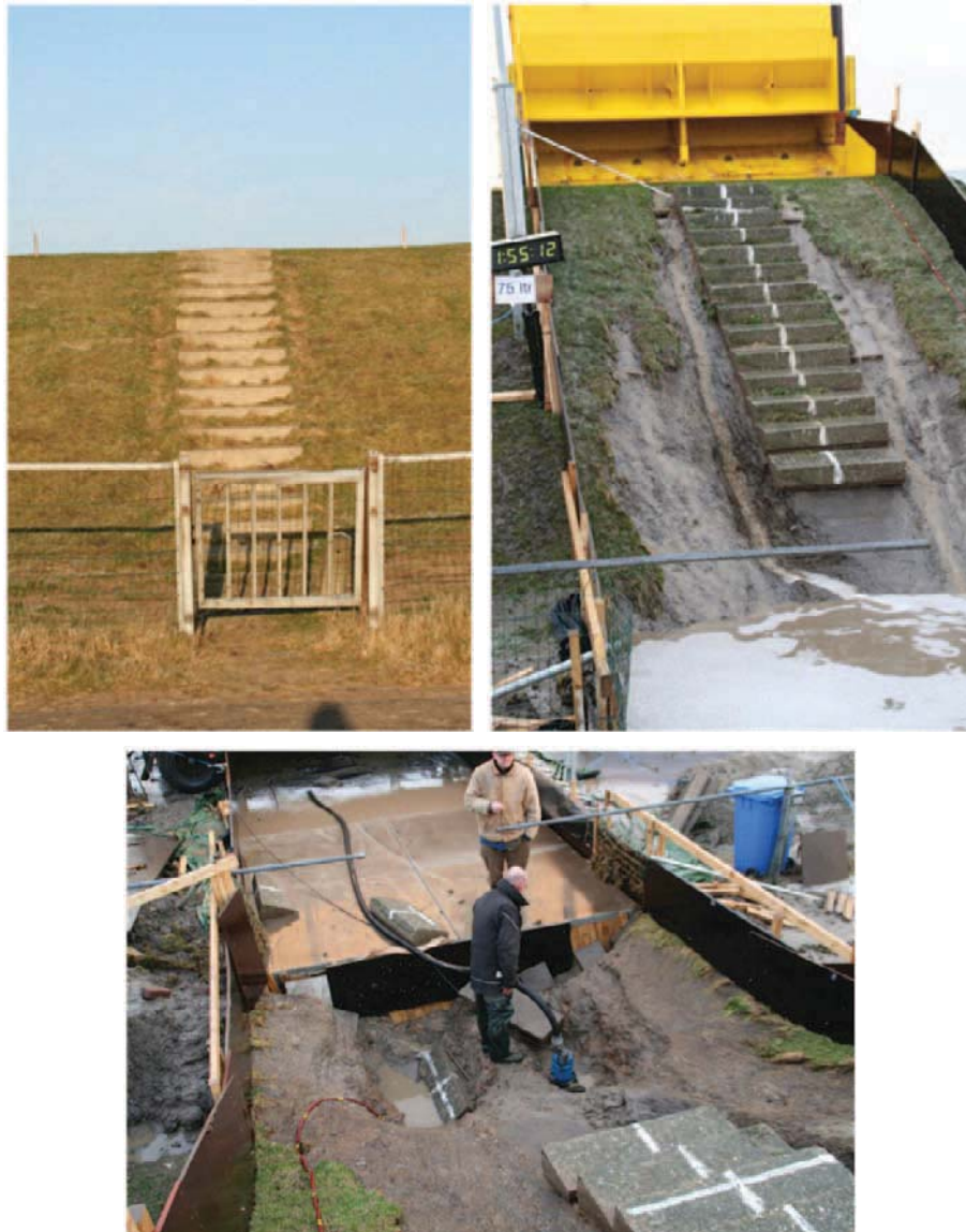
Figure 29: Afsluitdijk. Staircase with fence, before and after testing, section 3. Left: before testing and right: after 2 hours of 75 l/s per m. The concrete staircase is near failure. Grass ripped off the slope, but gully development occurred only along the staircase where concentration of flow was observed. Hardly damage to the clay layer. The brick path to the staircase was completely destroyed, as well as the fence gate. Two erosion holes developed at the toe, due to the concentrated flow along the staircase. Holes about 1 m deep, but not reaching the sand core (cover by 0.4 m clay and 1 m boulder clay). Situation after 2 hours of 75 l/s per m.
