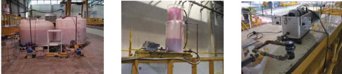
Figure 3: Tanks and hydraulic system (left and centre). Flow-meter and flow control valve (right)
