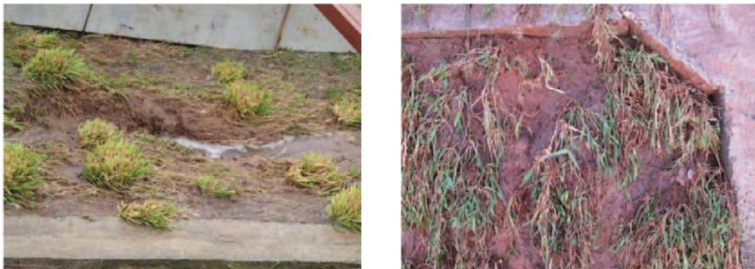
Figure 8: Left: damages amongst Vetiver clumps. Right: poor cover of Bermuda grass and settlement of soil around concrete beams,
