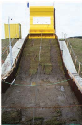
Figure 28: Afsluitdijk. Grass toe, section 1. Grass ripped off on many locations on the slope and completely at the horizontal part, where a section of 4x4 m 2 was created without grass. The good clay (still with roots) showed hardly any erosion and resisted without problems 75 l/s per m. Erosion holes near toe about 0.4 m deep.
