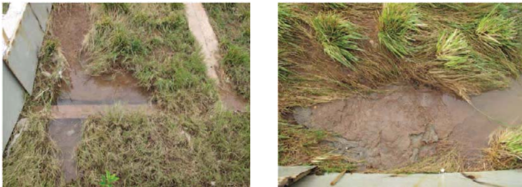
Figure 7: Left: concrete beam was exposed. Right: mortar layer under a top grass sod.
