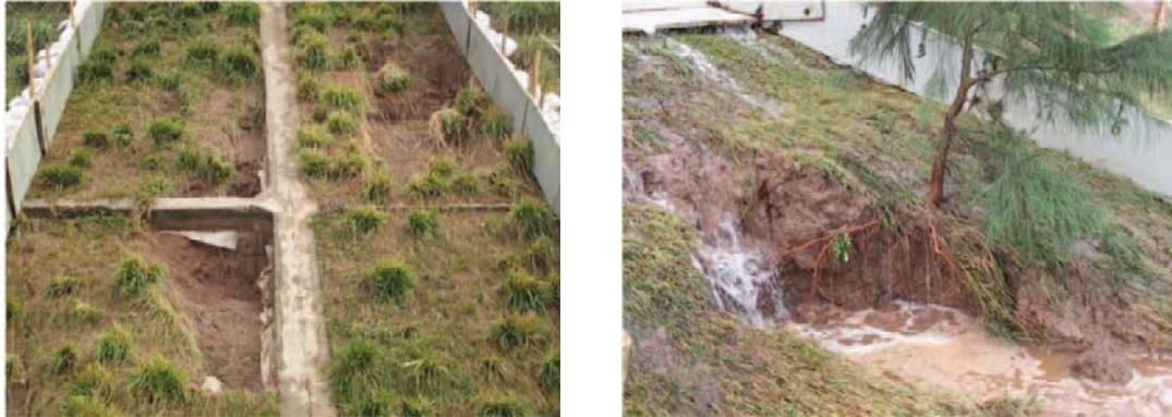
Figure 9: Left: damage around concrete frames. Right: damage extension to the Casuarina tree.
