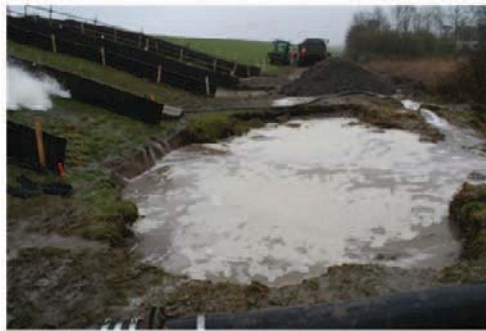
Figure 27: Kattendijke, Zeeland, section 1. Damage to the rear side at the maintenance road, which started at 30 l/s per m. Removal of the whole maintenance road. Picture taken half way the 75 l/s per m test. The hole became at the end 15 m wide and about 1 m deep.
