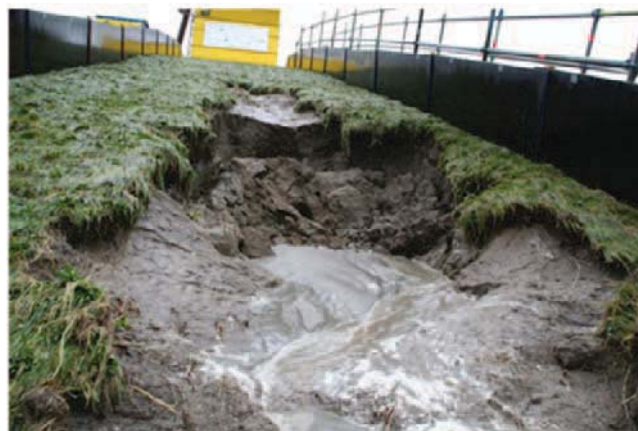
Figure 25: Final result Boonweg, Friesland; section 4. After 5 hours and 51 minutes with 75 l/s per m. The sand core has been eroded to at least 1 m depth and the right side wall is about to collapse. Final result about 45 minutes after first damage was observed.
