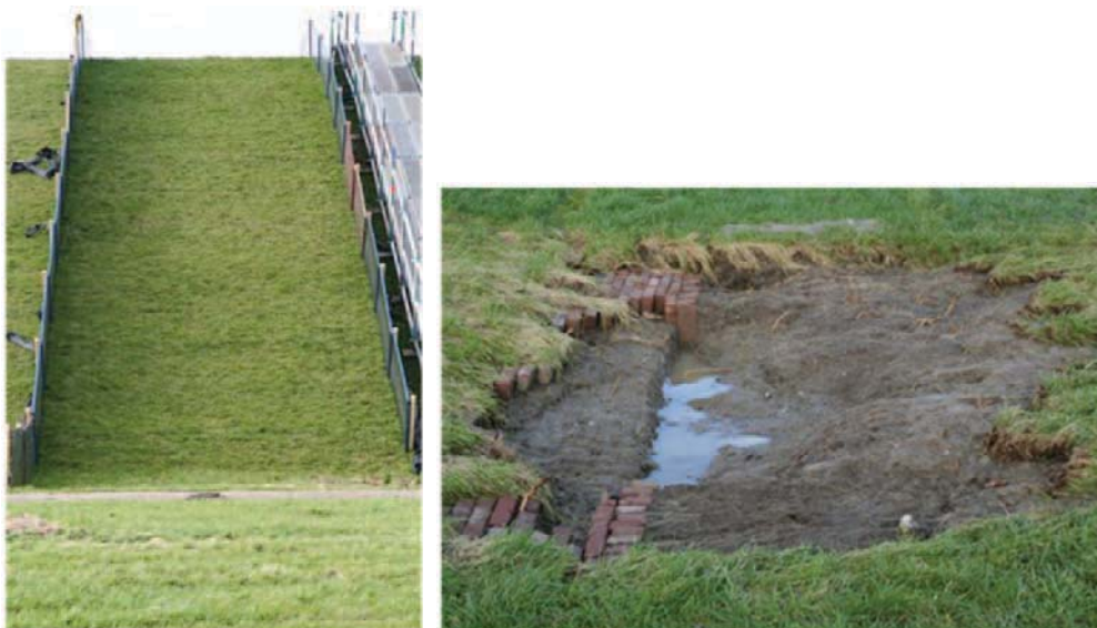
Figure 24: Final result Boonweg, Friesland, sections 1 and 2. No damage after 75 l/s per m. In the last hour of 75 l/s per m damage to the toe (hidden path of brick stone, see photo right).
