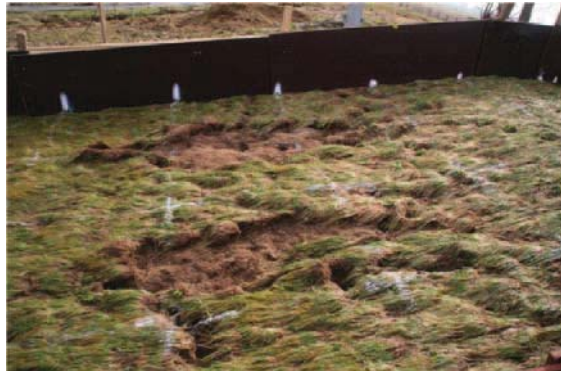
Figure 31: Various damaged locations.
