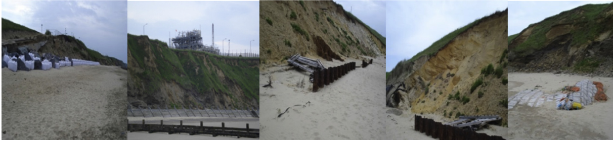
Fig. 4. Damage at the coastal front of the Bacton Terminal. Source: Bacton terminal operating company.
