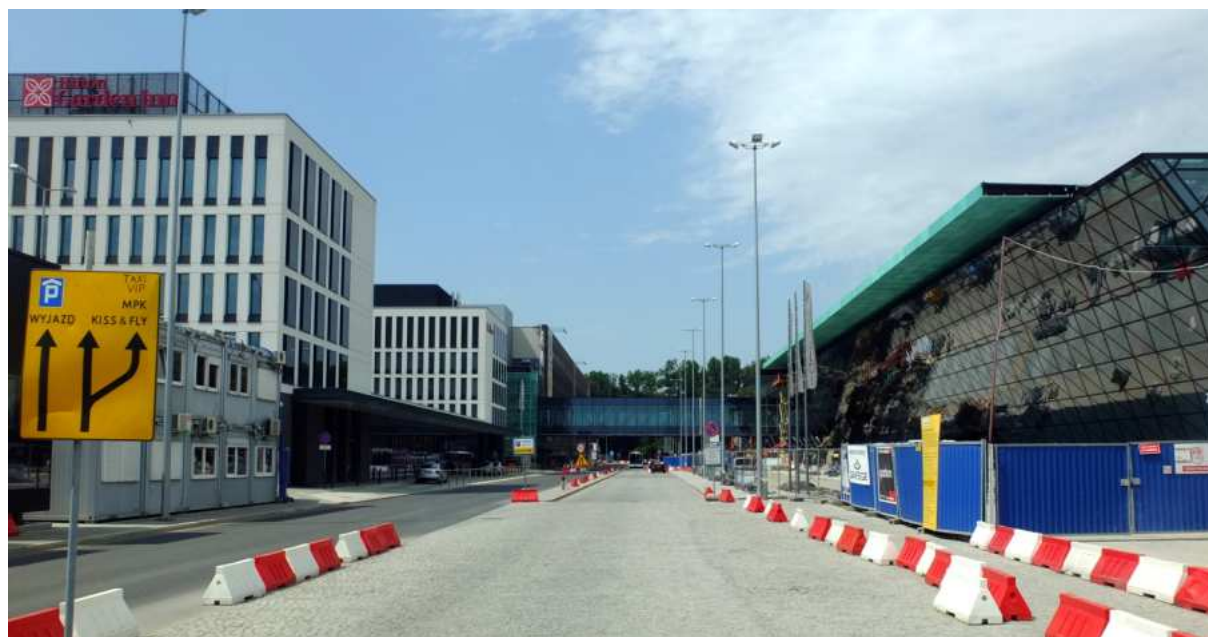
Figure 10. The street-like space in front of the extended terminal at Kraków Airport. Project by APA Czech Duliński Wróbel, under construction, July 2015 (fot. MS)
