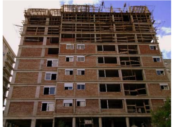
Figure 2 – Cooperative “COVIVEMA V”, first building over 5 floors under construction for mutual aid.
