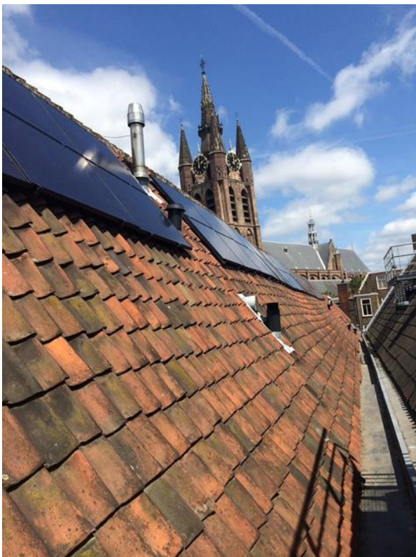
PV panels on the roof of Prinsenkwartier
