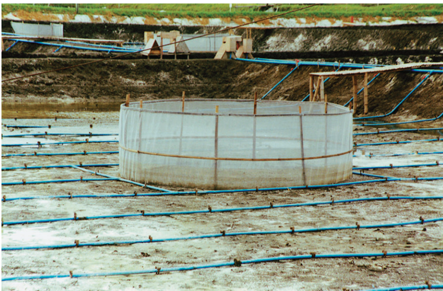
Fig. 12. Bottom aeration system with center sludge collector.
