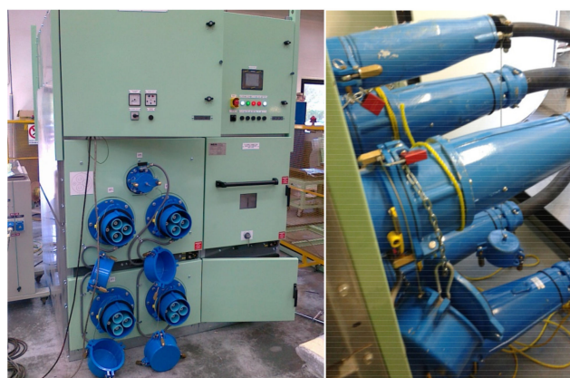
Figure 5. Switchboard for shore connection purposes [25].
