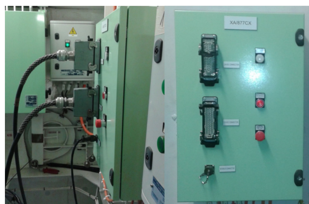
Figure 6. Shore connection control cabinet [25].
