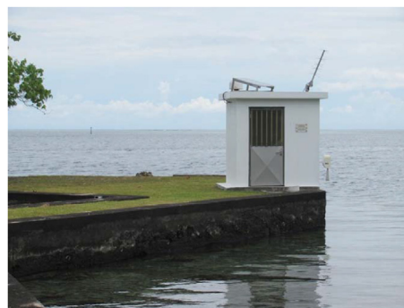
Fig. 2. The typical Tide Gauge geodetic station of Vairao (Tahitilti peninsula of Tahiti). One can see the RADAR altimeter (vertical corner on the right side), the GOES UHF Yagi antenna on the roof as well as the GPS radome and a solar panel.
