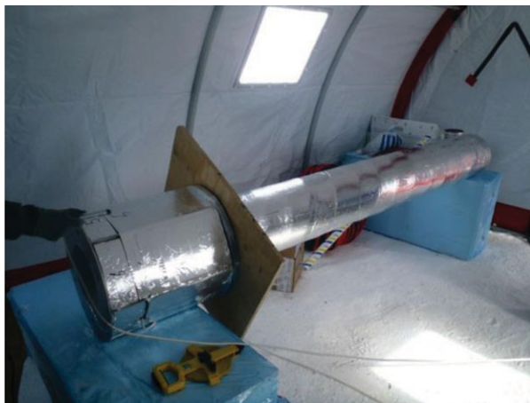
Figure 5. Photograph of the stainless steel wellhead section with heat trace and insulation applied. (Online version in colour.)
