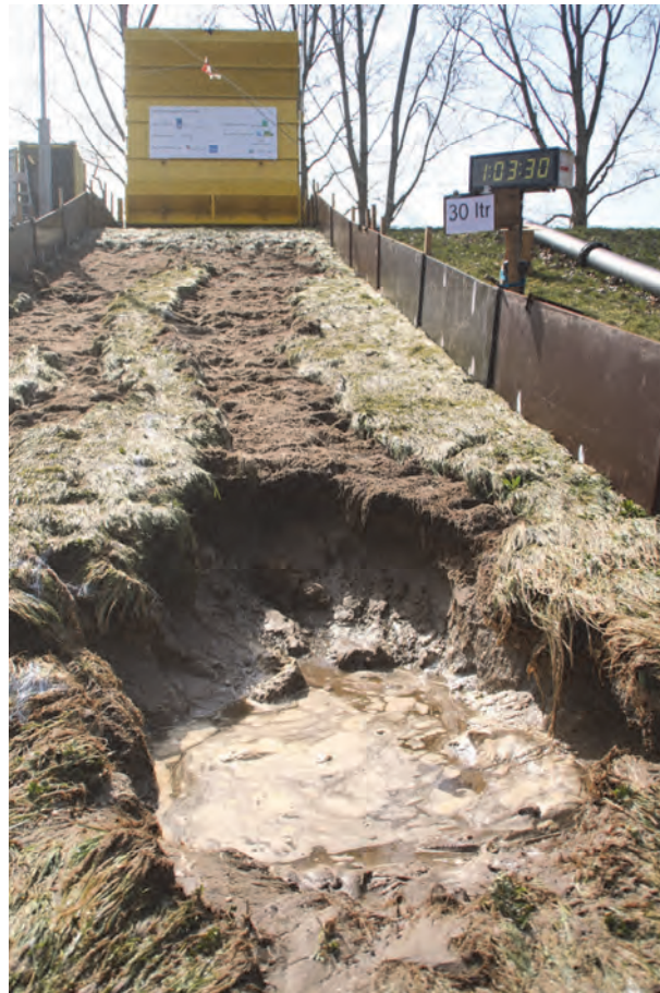
Figure 4.35 Failure of a grass covered sand dike
