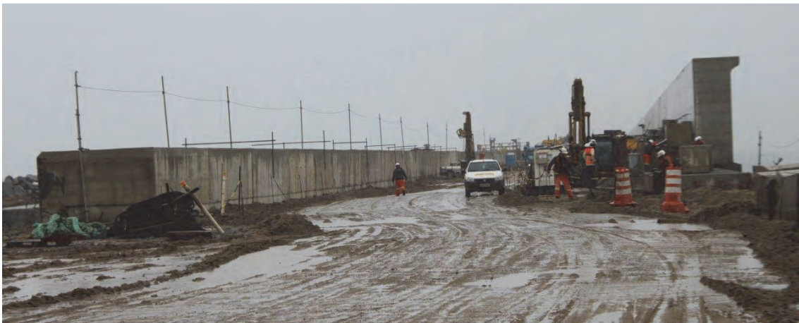
Figure 1.7: A relatively small bull nose on the crest wall of a large caisson. The caisson under construction, Açú, Brasil, is 25 m wide and the crest level is 10 m above sea level
