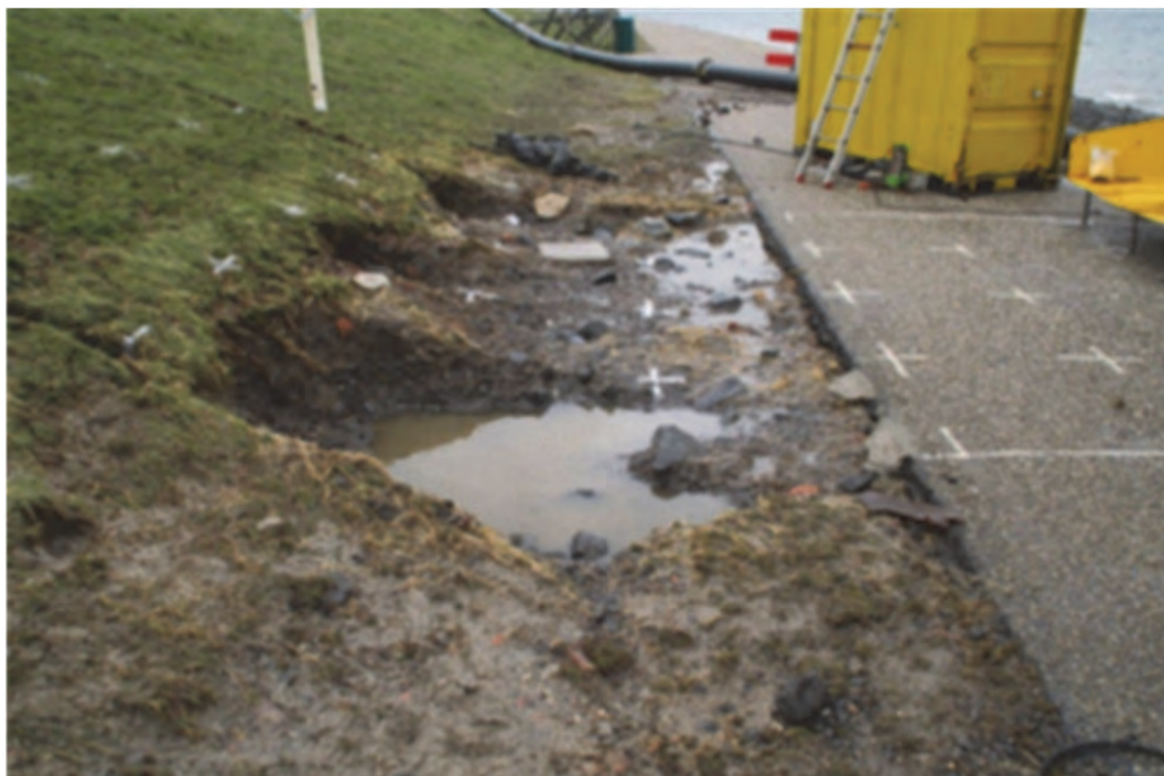
Figure 4.39 Final damage after the pilot run-up test
