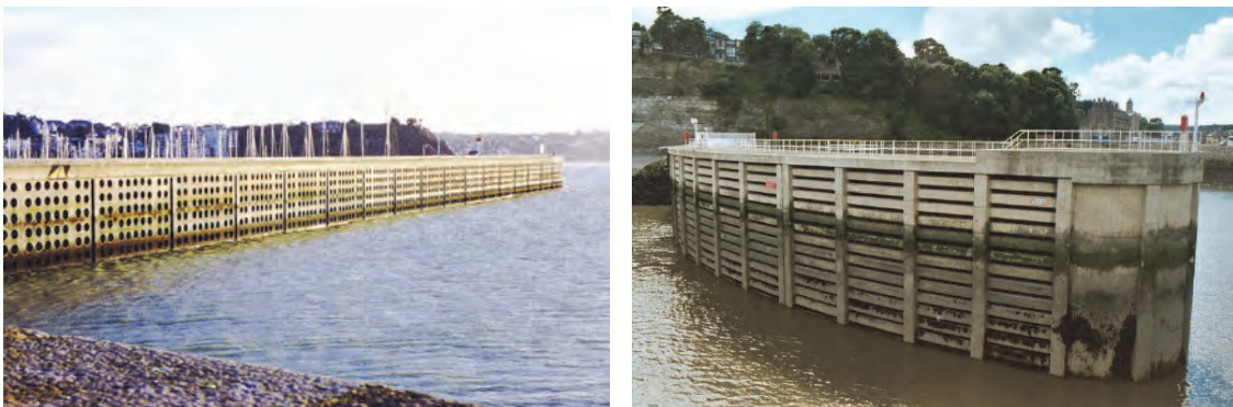
Figure 7.24: Examples of perforated caissons, left Caen, France and right Cardiff Barrage, UK
