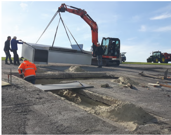
Figure 7.3: Excavation of the dike slope and placement of the overtopping tanks inside the dike.
