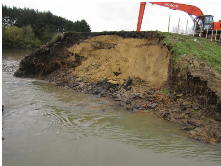
Figure 5-3 Breach during test II 17/11/2015
