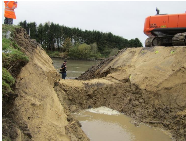
Figure 5-2 Breach after breach test I 16/11/2015
