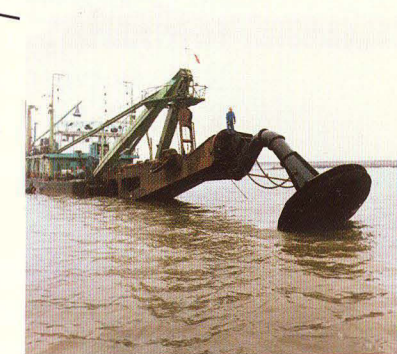
The diffuser for the environmentally friendly disposal, of dredged silt in underwater cells
