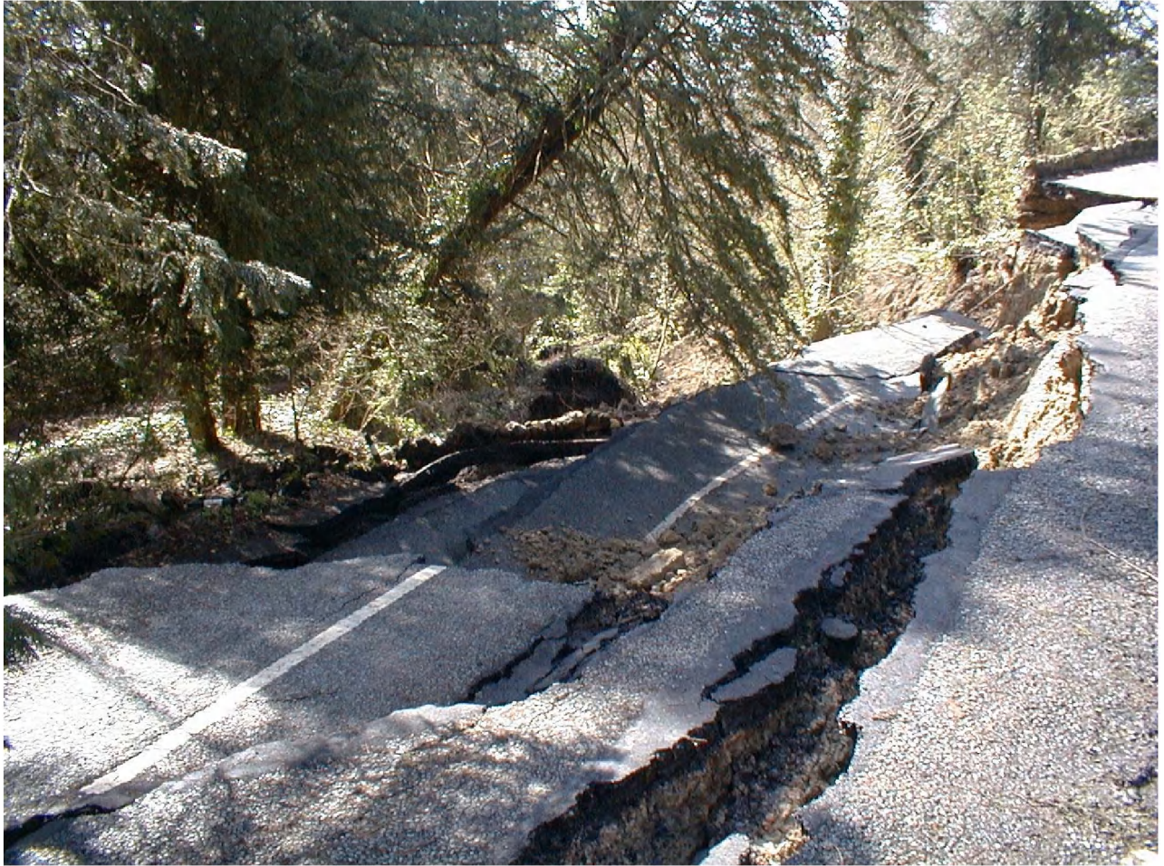
Failure of the A3055 coastal road in April 2001, near the town of Ventnor, Isle of Wight, UK, at the crest of a coastal mudslide (part of the important circular 'round the island' road).
