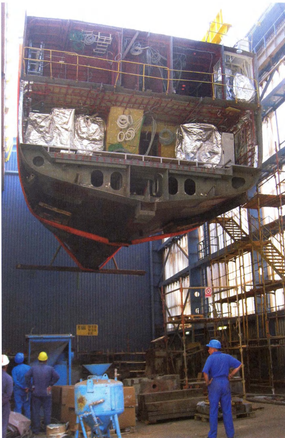
The hull construction and basic outfitting took place at Damen Shipyards Galati (Romania)
