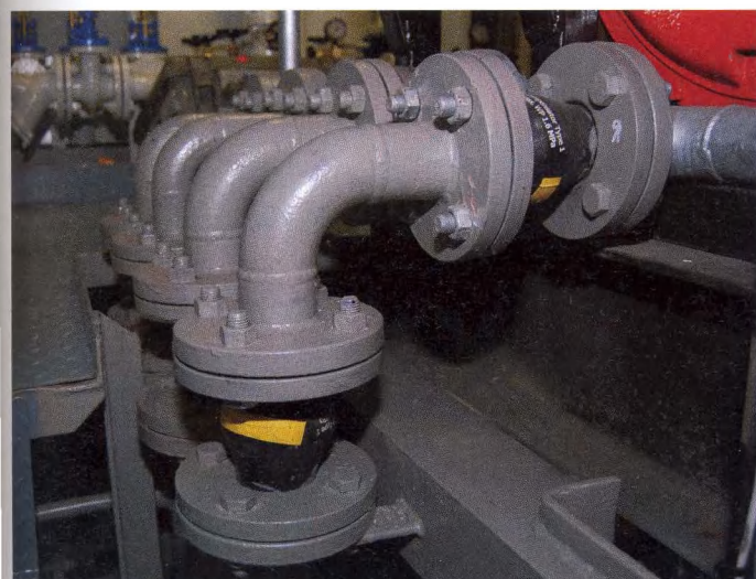
Piping leading to the gensets have bellows in two directions to eliminate the transfer of vibrations
