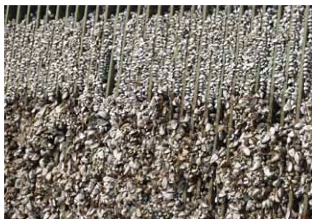
The zebra mussel can cause damage by blocking pipes, vents and any holes or openings where water flows. Reservoir tower safety grating clogged with zebra mussels (Rabisha Reservoir, Bulgaria).
