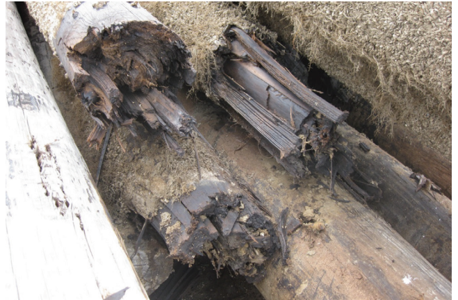
Figure 4: Broken pile fractured ends
