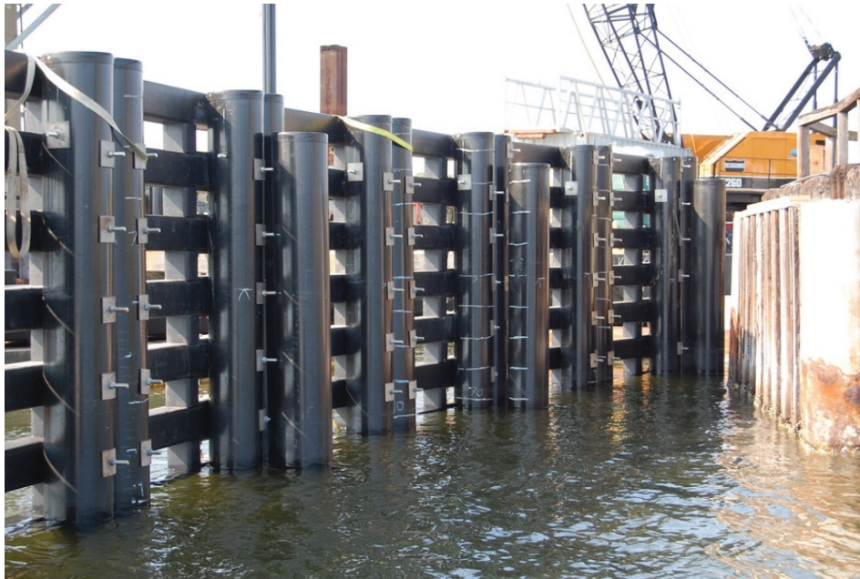
Figure 5: Example of hollow composite pile in small clusters with composite timber walers
