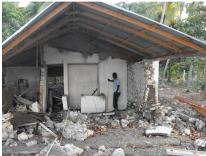
Figure 3. High water mark in house (Photo: Hermann Fritz)
