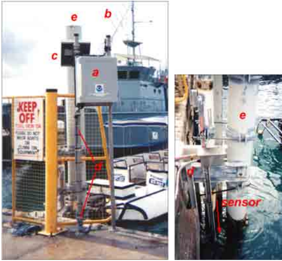
Rarotonga sea level station, Avarua Harbor, Cook Islands. The fiberglass electronics package (a), antenna (b), solar panel (c) were installed on a pier. Conduit (d) containing cables connecting the sensor, located at a depth of five feet below low-tide water level, to the data collection platform containing the electronics above, was externally attached to the tube containing the sensor (e).
