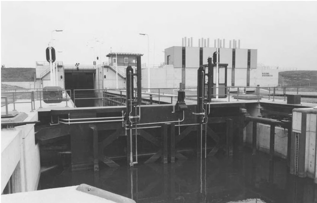
Photo 7.33 Hydraulic cylinder lock paddle operating mechanism of a single pivot gate of the lock at Nieuwe Statenzijl
