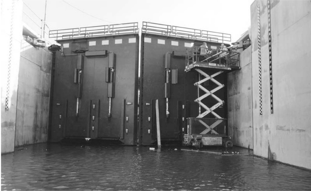
Photo 6.10 Lock paddles for the rectangular openings of the mitre gates of the Kleine Sluis in IJmuiden
