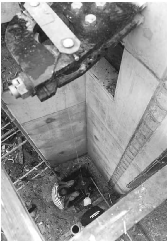
Photo 7.13 Adjusting the pivot of a single pivot gate of the lock in Gorinchem (1987)
