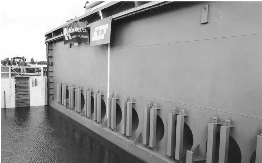
Photo 6.13 Energy dissipating bars behind the round openings of the sliding gate of Nieuwe Oranje lock in Amsterdam
