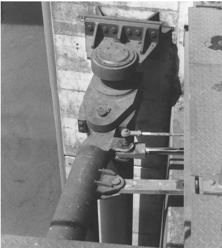
Photo 7.22 Detail of the locking device for single pivot gate of the lock at Nieuwe Statenzijl
