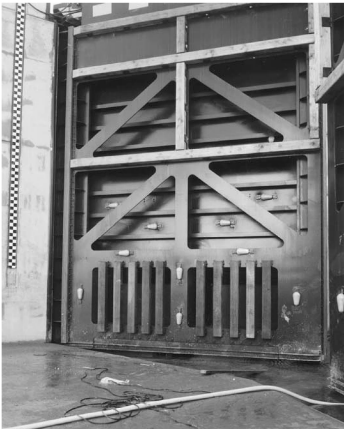
Photo 6.11 Energy dissipating bars behind the rectangular openings of the mitre gates of Kleine Sluis in IJmuiden
