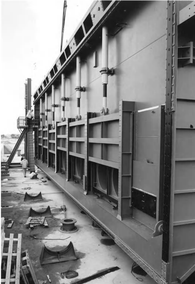
Photo 6.12 Sluice gates in front of the round openings of the sliding gate of Nieuwe Oranje lock in Amsterdam
