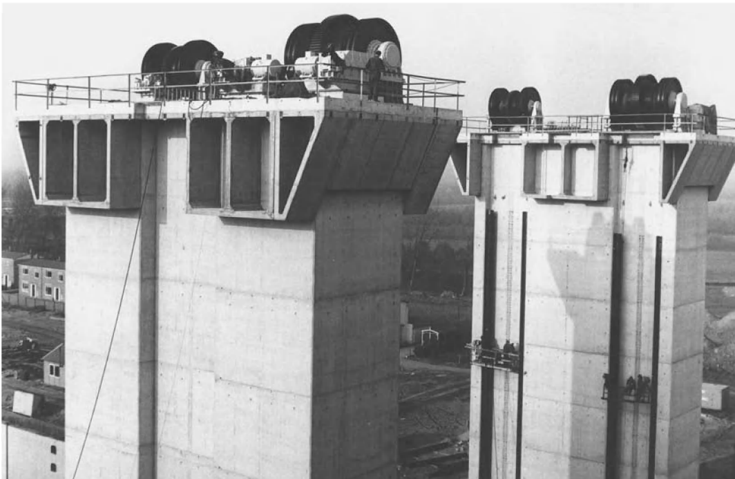
Photo 7.31 Operating mechanism of the lift gate of the new lock in Wijk bij Duurstede
