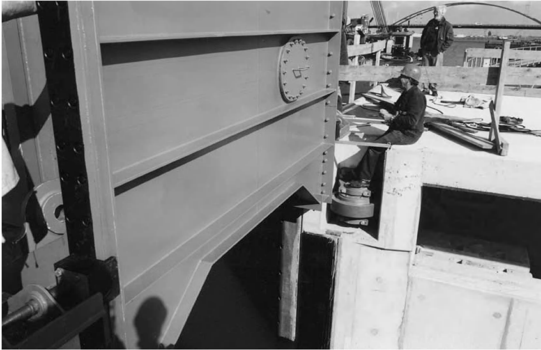
Photo 7.30 Horizontal guide wheel of the sliding gate at Nieuwe Oranjesluis in Amsterdam
