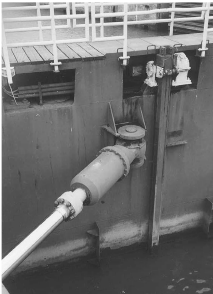
Photo 7.19 Hydraulic cylinder gate operating mechanism and direct rack bar and lock paddle operating mechanism of push-tow locks in the Volkerak
