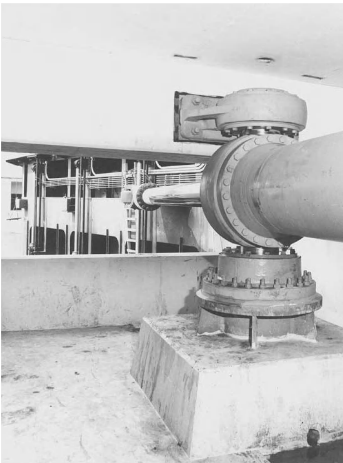
Photo 7.18 Hydraulic cylinder gate operating movement at Rozenburgse lock
