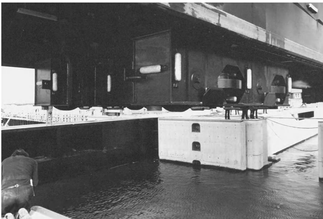
Photo 7.27 Lower roller carriage of the rolling gate at Middelsluis in Terneuzen
