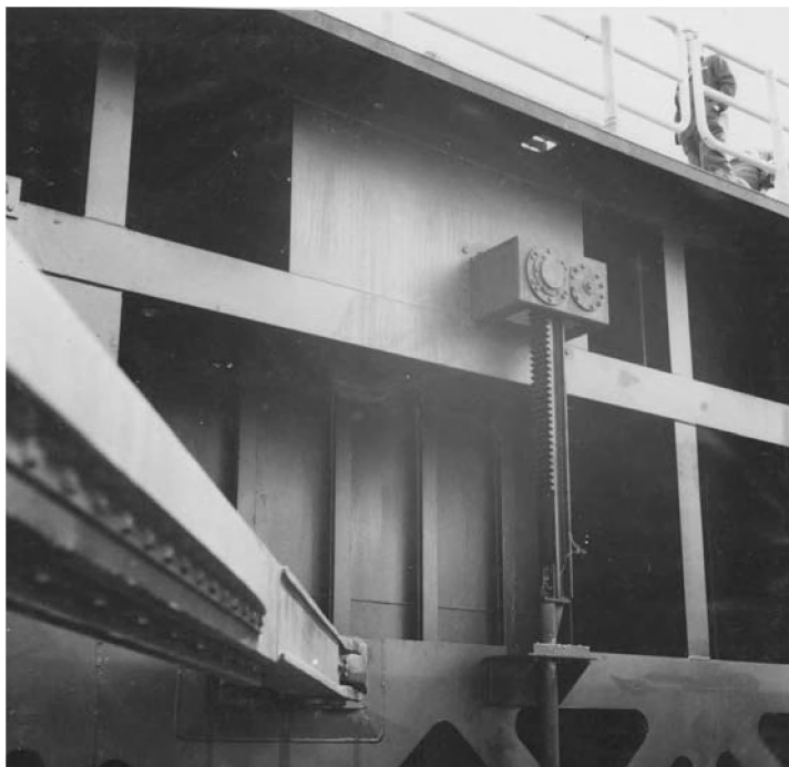
Photo 7.15 Direct rack bar for gate and sluice movement of Koopvaardersschutsluis in Den Helder
