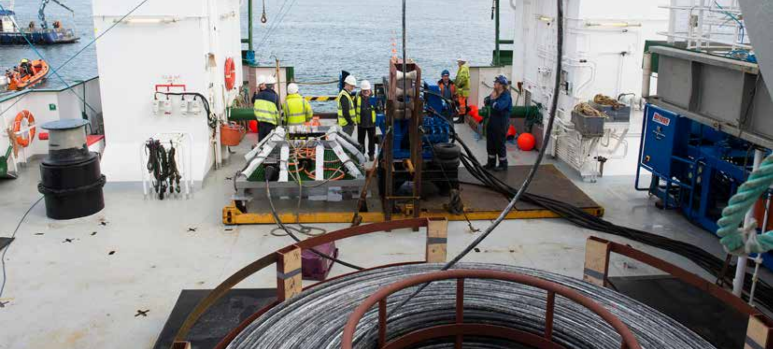
Fibre optic and power cable installation at the Galway Bay test site, Ireland
