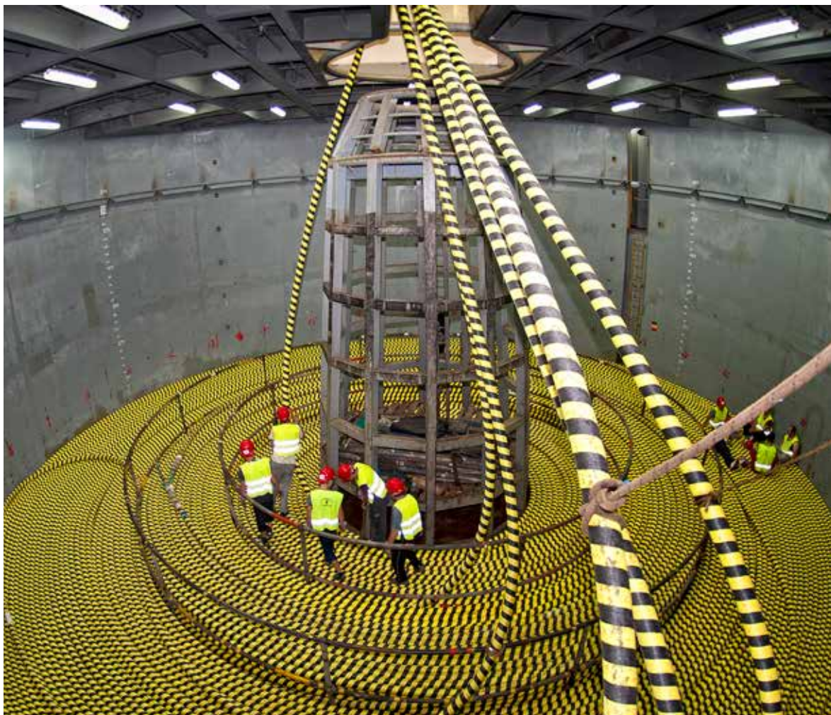
Power cable drum housing at the European Marine Energy Centre, Scotland
