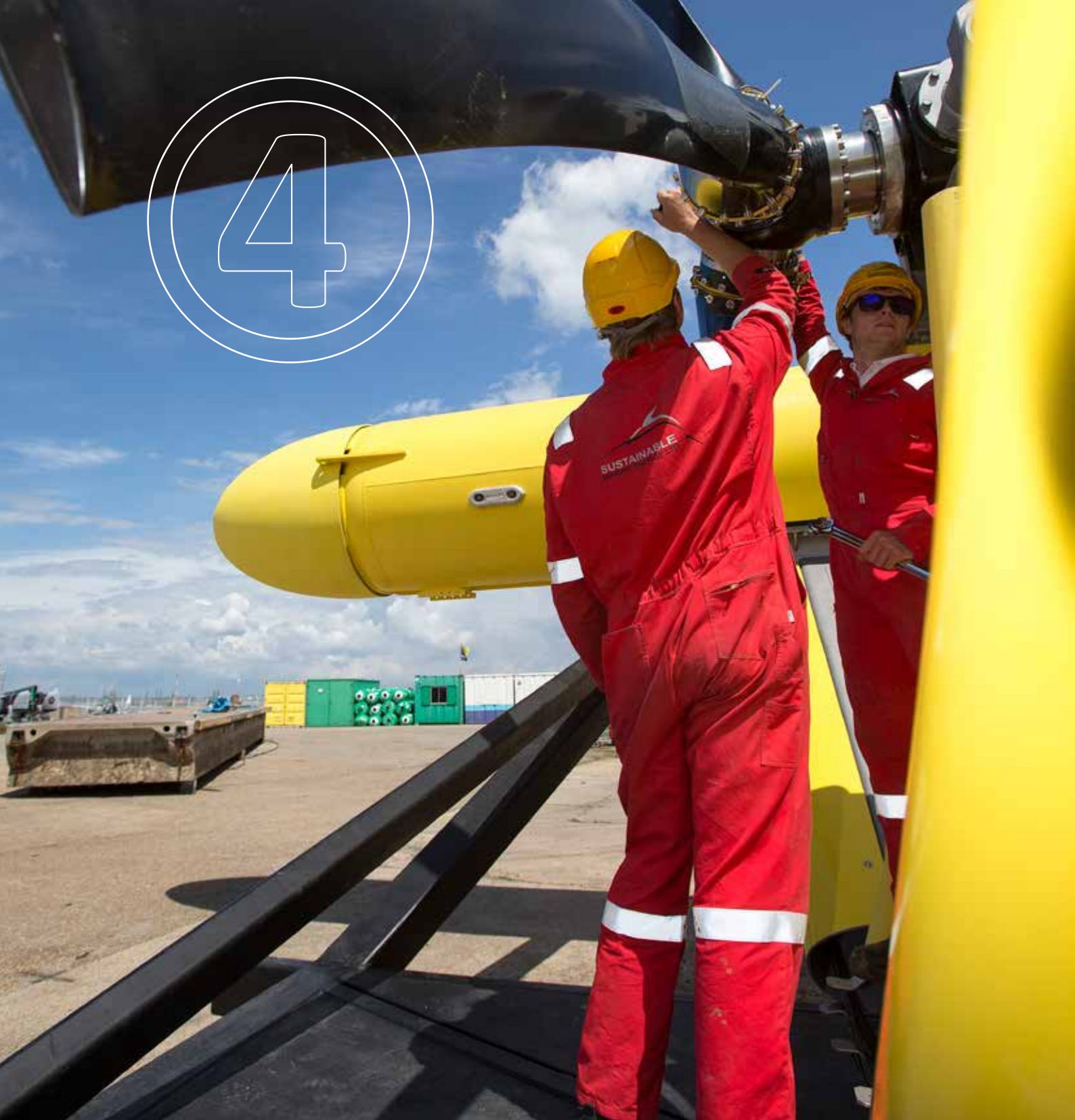
Schottel Hydro SIT turbines loaded onto a Plat-o tidal platform
