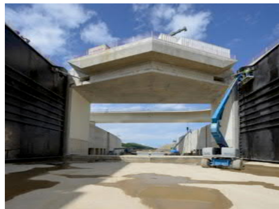
Fig.6: Downstream mitre gate – © JL DERU/photo-daylight
