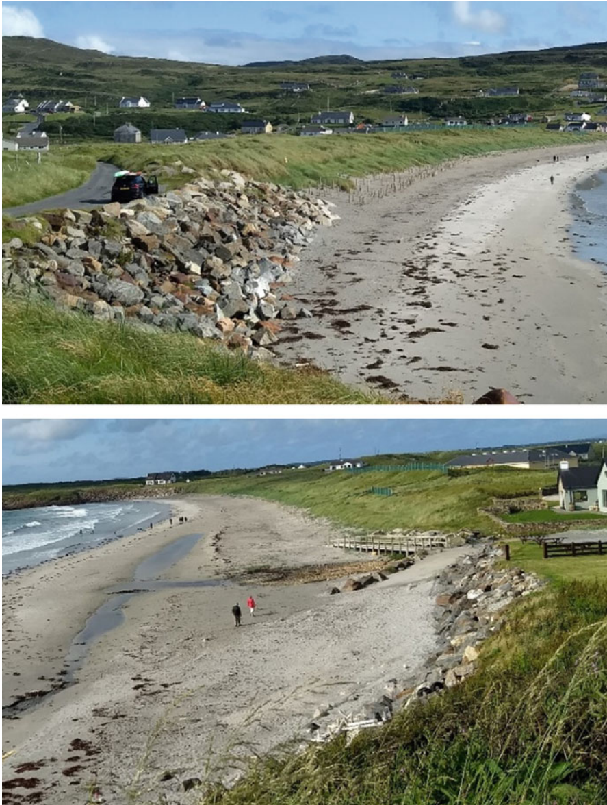
Fig. 32.2 Rock Armour on the northern and southern sides of the beach. (Photo: Paul Lawlor, 2019)
