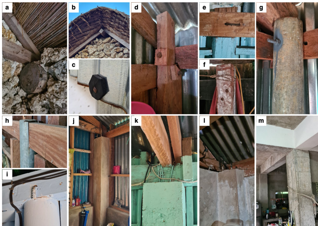
Figure 3. Structural details documented across the typologies surveyed. (a) Roof-to-wall connection where thick logs are embedded in stone walls and (b) layered thatch (cogon) roofing with reed matting are features of URM. (c) Improvised rubber washers for nail fasteners are used for typologies with CGI sheets. For LW-A, common post-and-beam connections are (d) bolted, (e) hooked with reinforcing steel bars, and (f) nailed. For LW-B and SC-A, common post-and-beam connections are (g) bolted, (h) notched and clipped, and (i) hooked with reinforcing steel bars. For SC-B, typical post-and-beam connections are (j, k) dowels wrapped around beams and roof members. For RC-A, (l) roof-to-wall connections are common to be via dowels from reinforcing steel bars wrapping the wooden roof members. For RC-B, (m) beams and columns are reinforced concrete supporting the slab roof.
