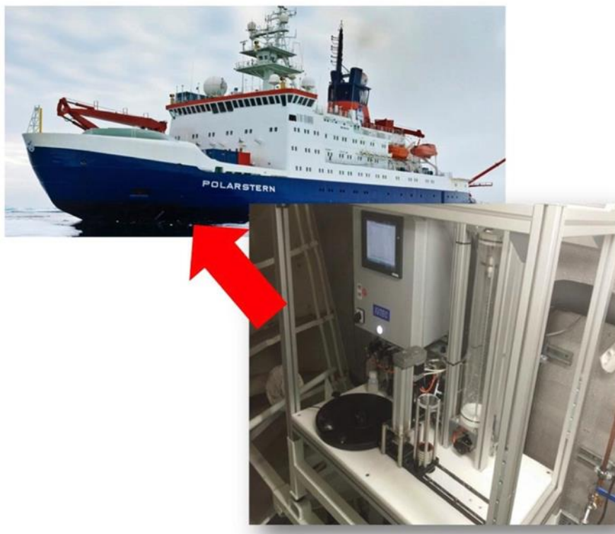
Fig. 3.1: The fully automated filtration module AUTOFIM is installed on RV Polarstern in the “Bugstrahlruderraum” close to the inflow of the ships-pump system. AUTOFIM is suitable for collecting samples with a maximum volume of 5 Liters. Filtration can be triggered on-demand or after fixed intervals. PHOTO: Katja Metfies
