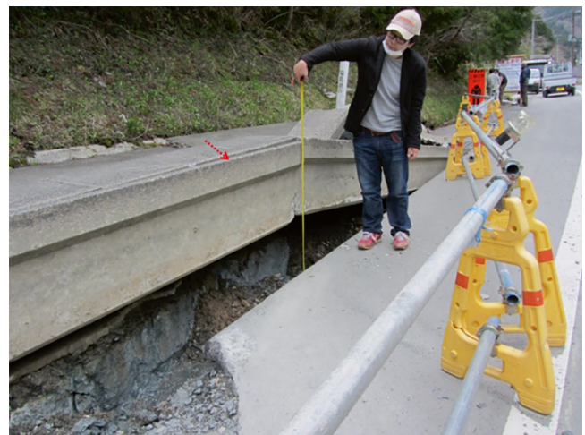
Fig. 6 Photograph rupture at junction of Highways 71 and 34, location c in Fig. 2
