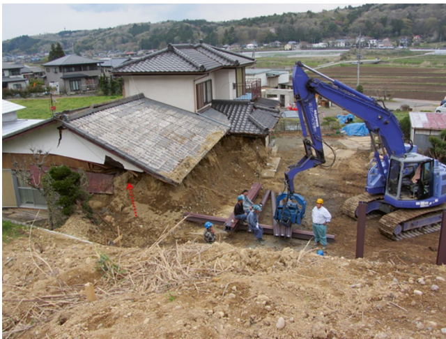
Fig. 19 A house filled with landslide debris at Kanaya Landslide
