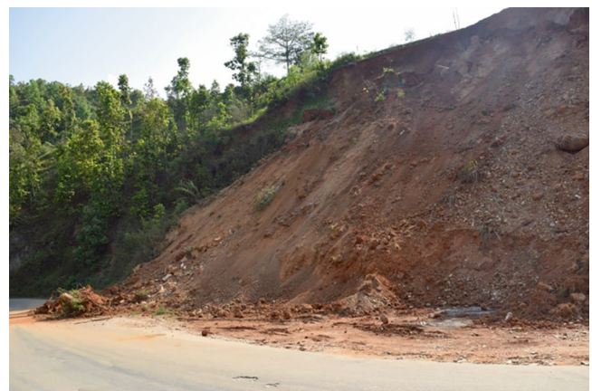
Fig. 53 Typical co-seismic landslide along the Araniko Highway
