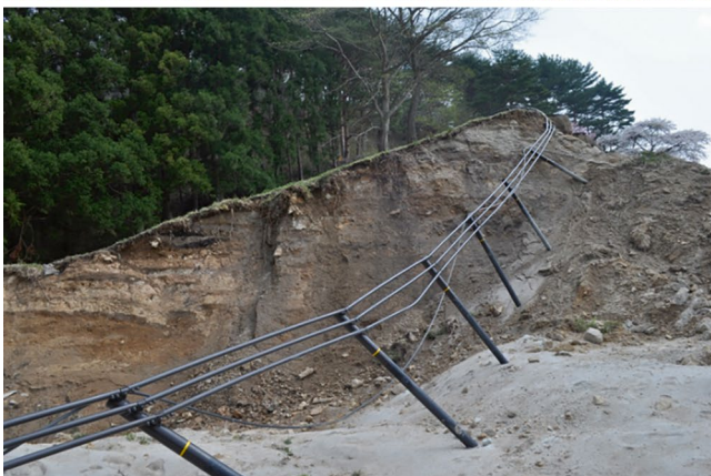
Fig. 48 Collapsed main dam portion of the Fujinuma Dam after the earthquake
