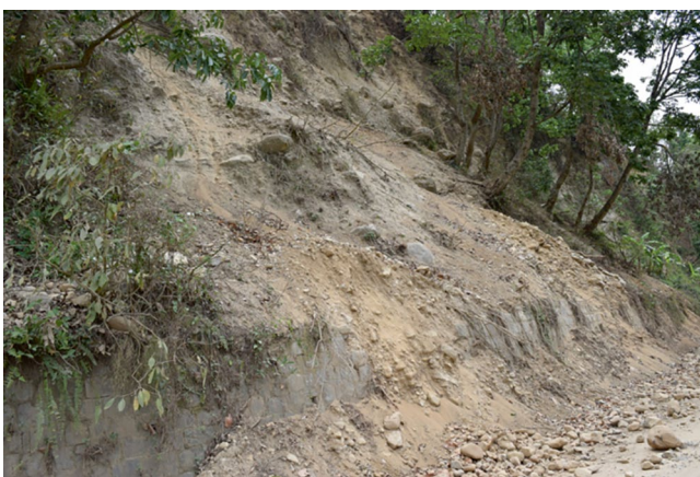
Fig. 60 Typical rockfall that blocked Melamchi Road at multiple locations
