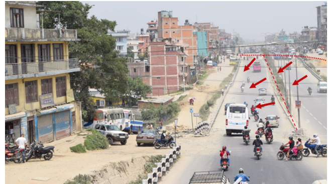
Fig. 89 Deformation of Araniko Highway at Lokanthali due to Gorkha Earthquake
