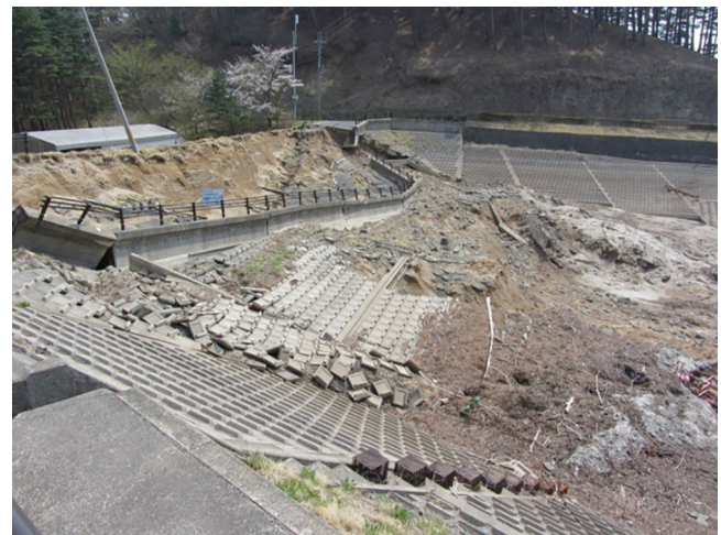
Fig. 49 Collapsed saddle dam portion of the Fujinuma Dam after the earthquake
