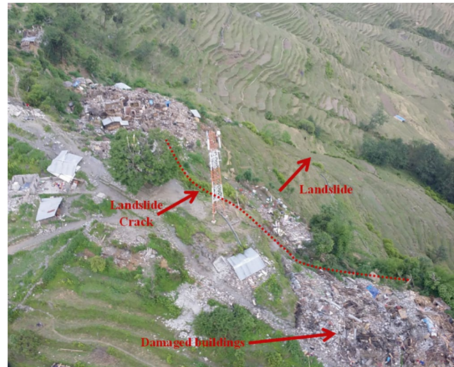
Fig. 88 Several long landslide scarps observed at the ridge above Barpak after the 2015 Gorkha Earthquake
