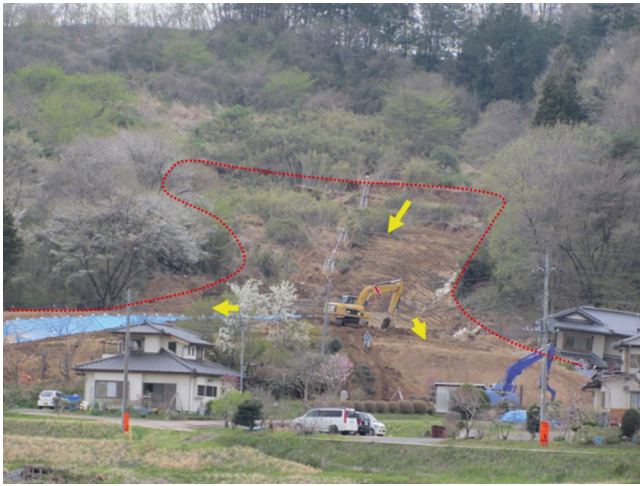
Fig. 18 Overall view of Kanaya Landslide from the toe
