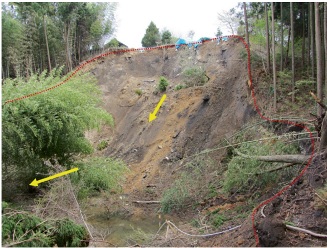
Fig. 31 Landslide damage at location ID 1 in the Kashiwazaki Residential Area
