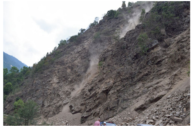
Fig. 61 Fresh rockfall observed at the Melamchi Access Road during field visit
