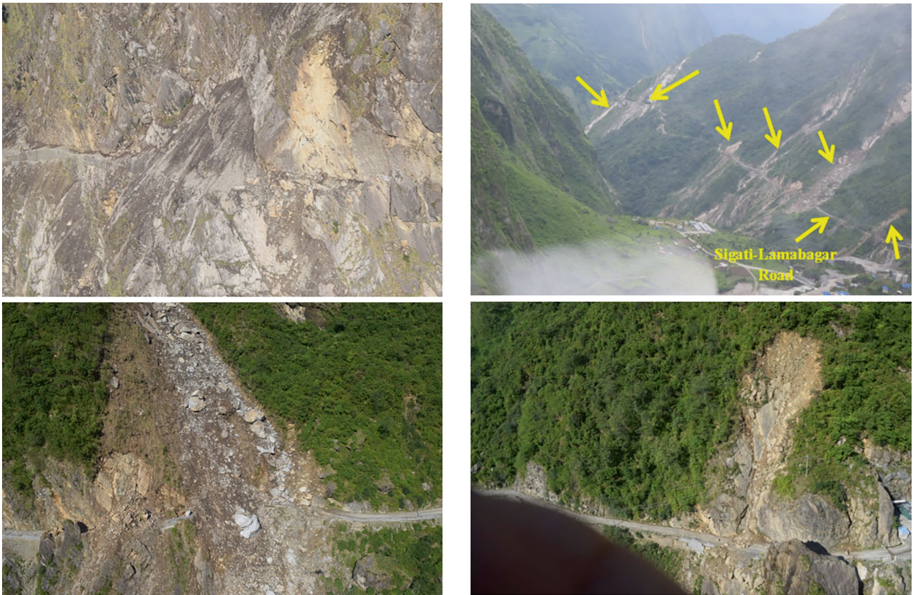
Fig. 62 Damages sustained by the Upper Tamakoshi Hydropower Project Access Road due to the 2015 Gorkha Earthquake
