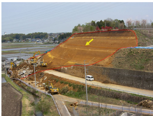
Fig. 15 Landslide that occurred at Gosaisho Highway
