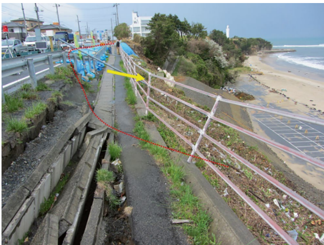
Fig. 44 Coastal landslide observed near Hitachi Bay
