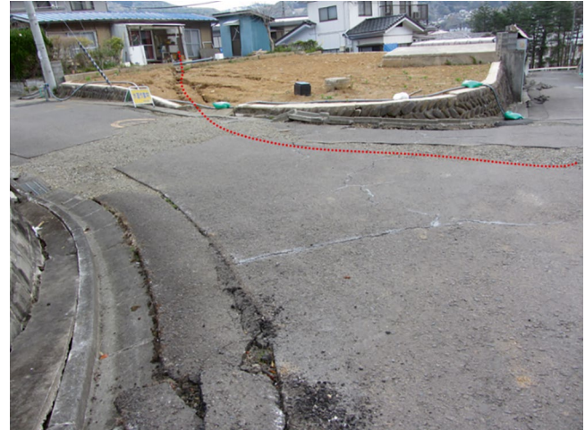
Fig. 34 Cracks on the road surface (location a) at Oritate Residential Area
