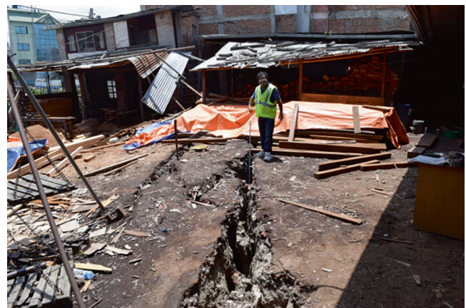
Fig. 90 Cracks observed along the Lokanthali ground failure area
