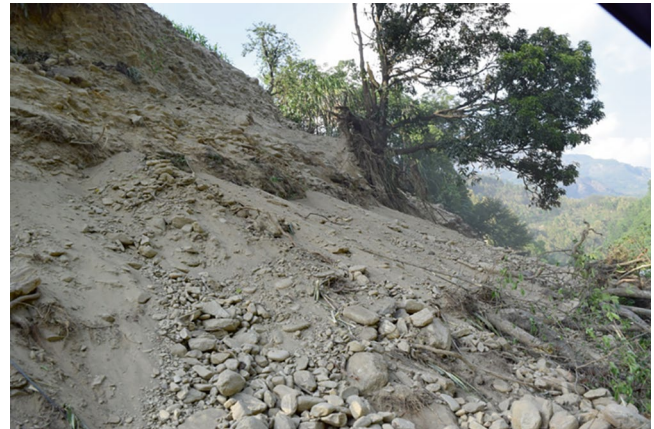
Fig. 56 Typical joint plane failure that threatened to block the Araniko Highway
