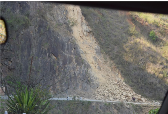
Fig. 54 Typical disrupted landslides that blocked the Araniko Highway at multiple locations
