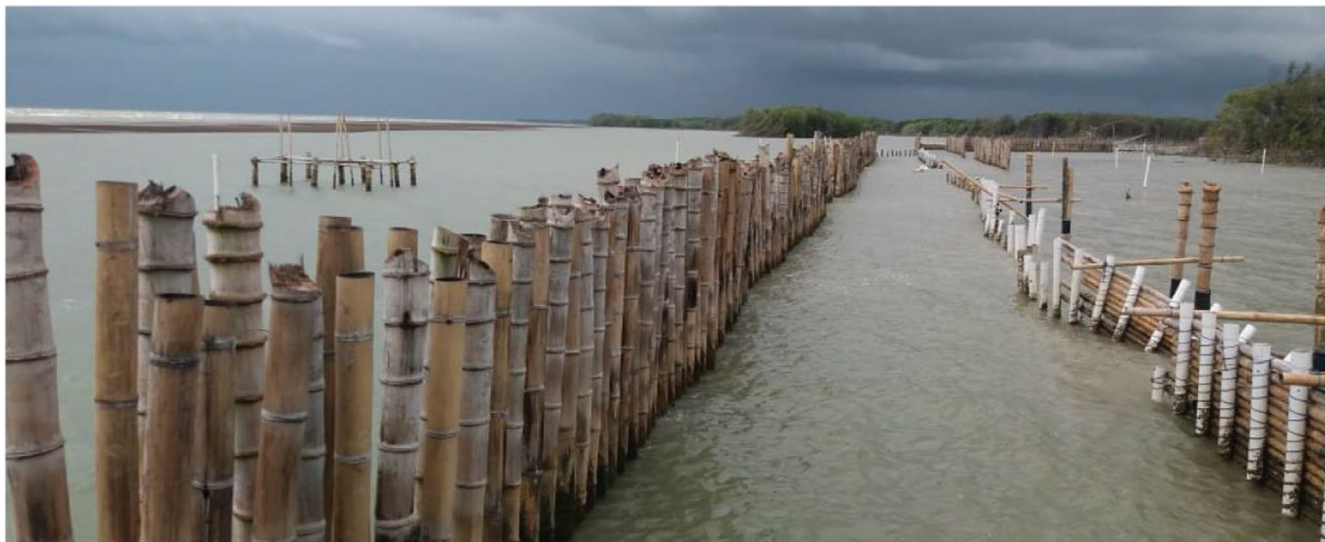
FIGURE 1 | Bamboo poles in support of coastal protection in Demak, Java, Indonesia, as part of the MuMaCo project. The semi-permeable structure functions as a wave barrier and consists of five elements, each 35 m wide, with a 5 m gap in between. Photo credit: Wawan Nugroho.
