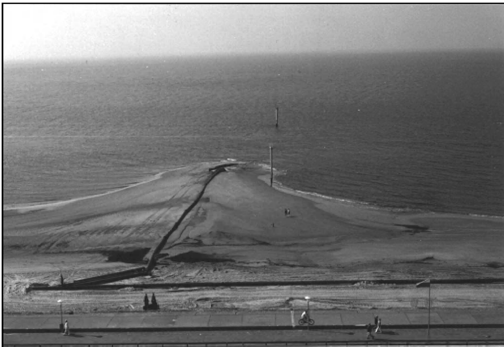
Figure 2. Execution of the shoreface nourishment by pumping humps of sand from the shore
