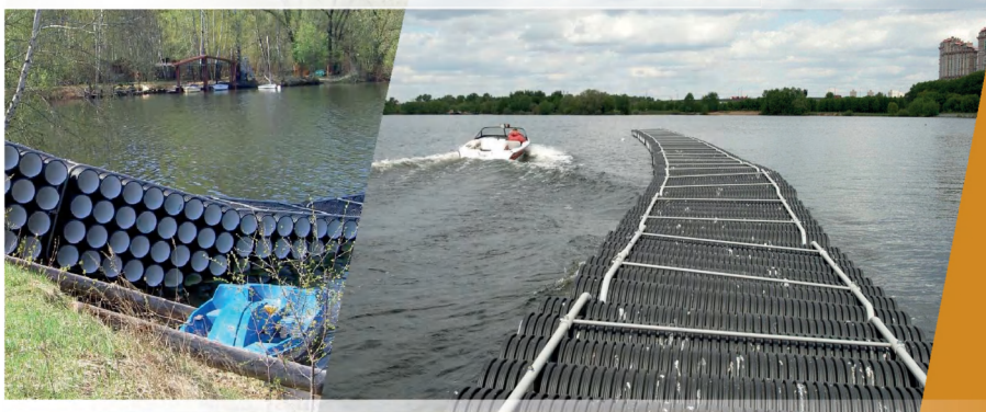
Floating breakwater made from plastic pipes can be used to protect against waves from recreational vessels (Copyright Kuznetsov).
