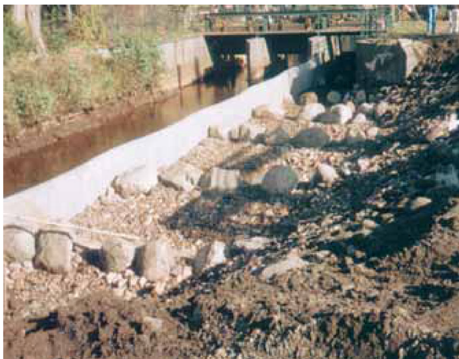
Figure 4.36: Delmenhorst fish ramp.
