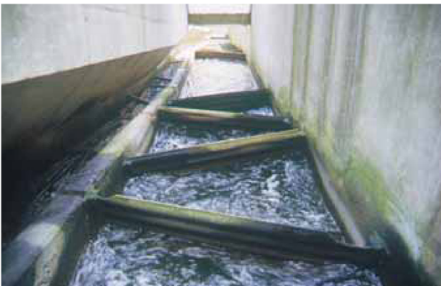
Figure 5.40: Rhomboid pass and eel ladder on the Sauer dam at Rosport (Rhineland-Palatinate). View from headwater.
